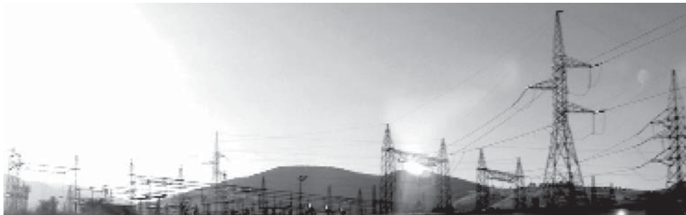
High voltage power lines and pylons
